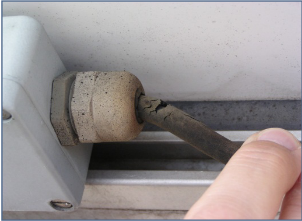
Cable overheating effect
