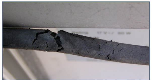
Ozone damage effect
