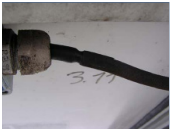
Installation misuse - violent pressure
