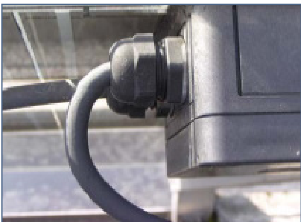
Cable handling misuse - bending radius too small
